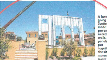
A $1.7 million home is going up in north Scottsdale's Silverleaf community using pre-engineered, factory-built steel walls.
